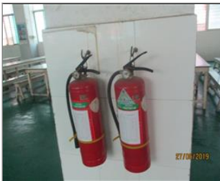
Photo of fire safety equipment Fire extinguishers.JPG
