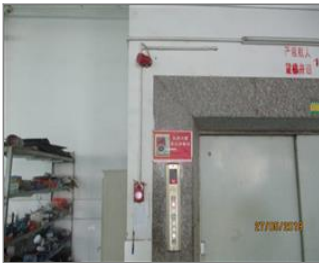
Photo of fire safety equipment Fire alarm.JPG
